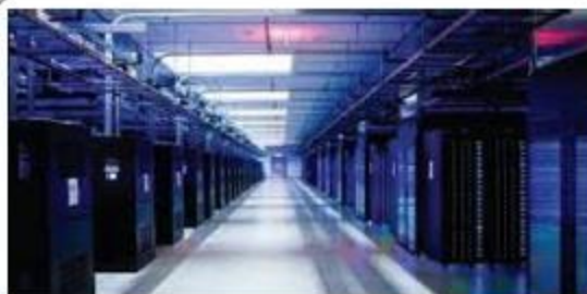
Smart Data Center
